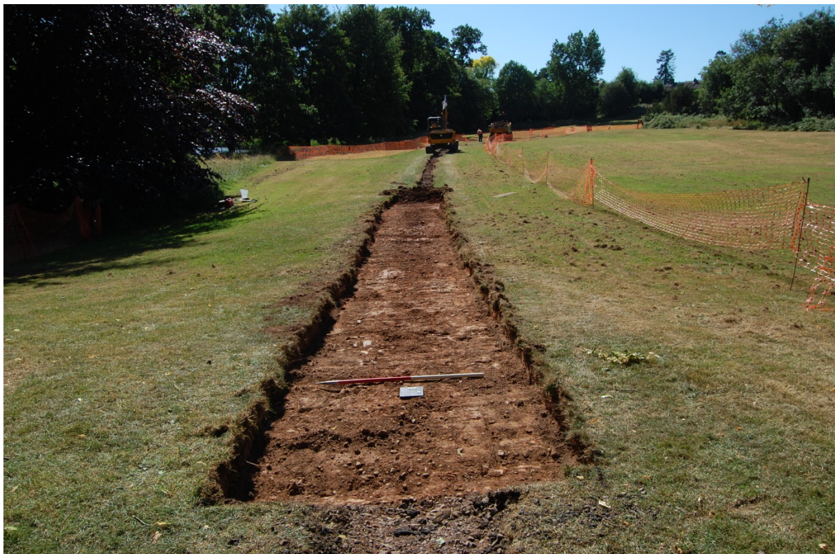
2: Stripping of topsoil and subsoil with a toothless bucket following removal of existing tarmac path
