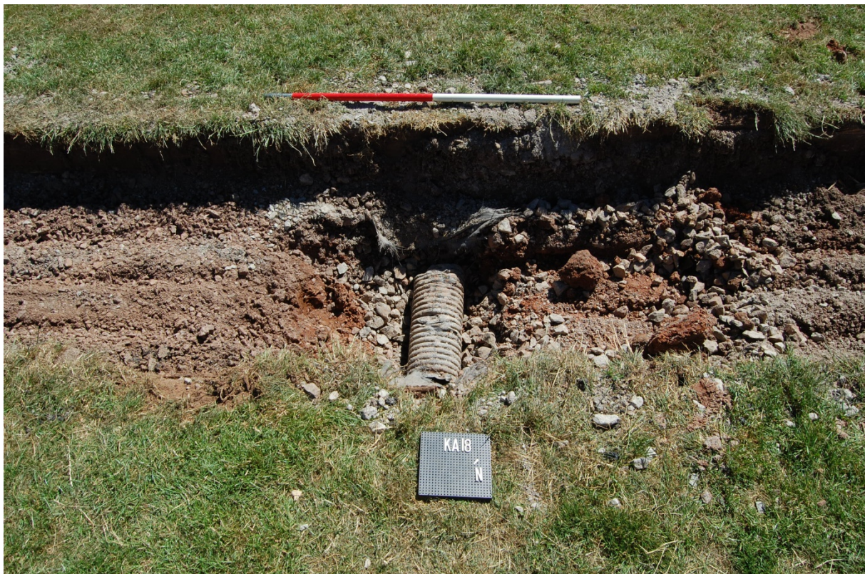
20: Modern plastic land drain revealed in the trench base following removal of modern tarmac path, looking south-east
