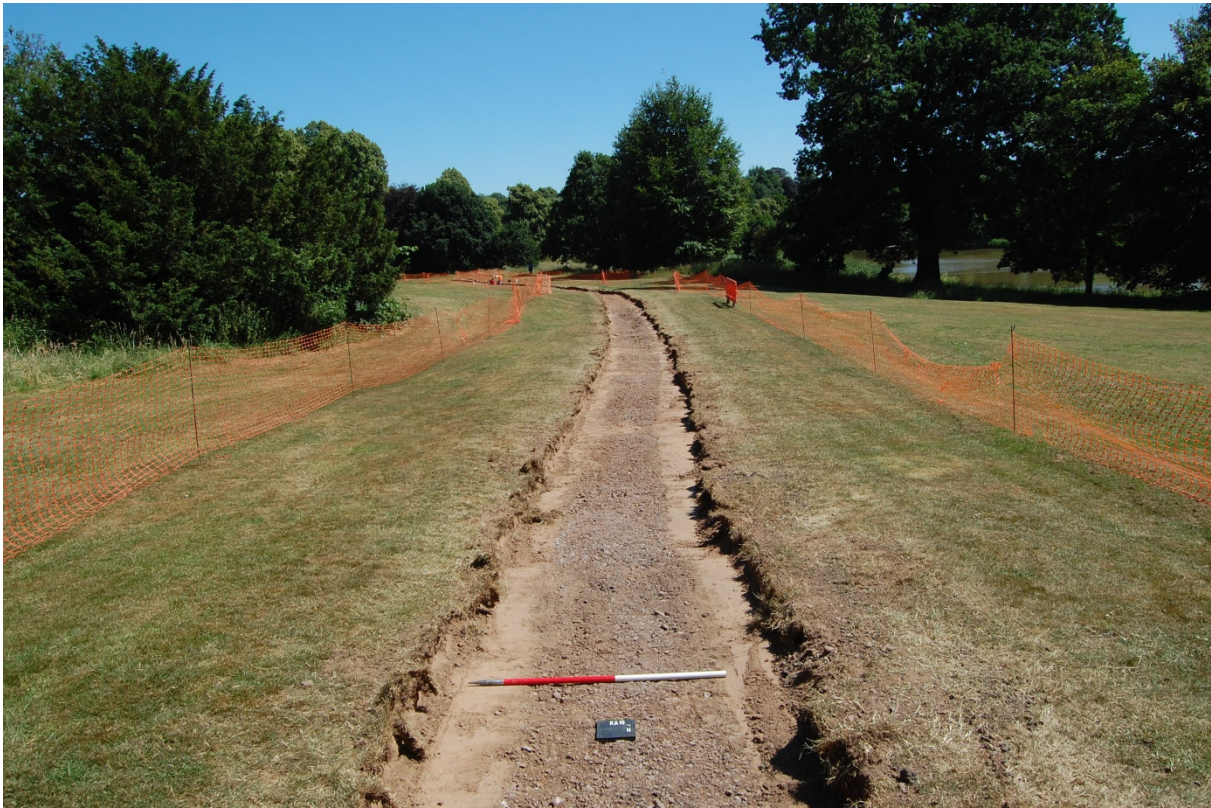
3: Trench for new footpath excavated to a depth of 0.25m with a toothless ditching bucket
