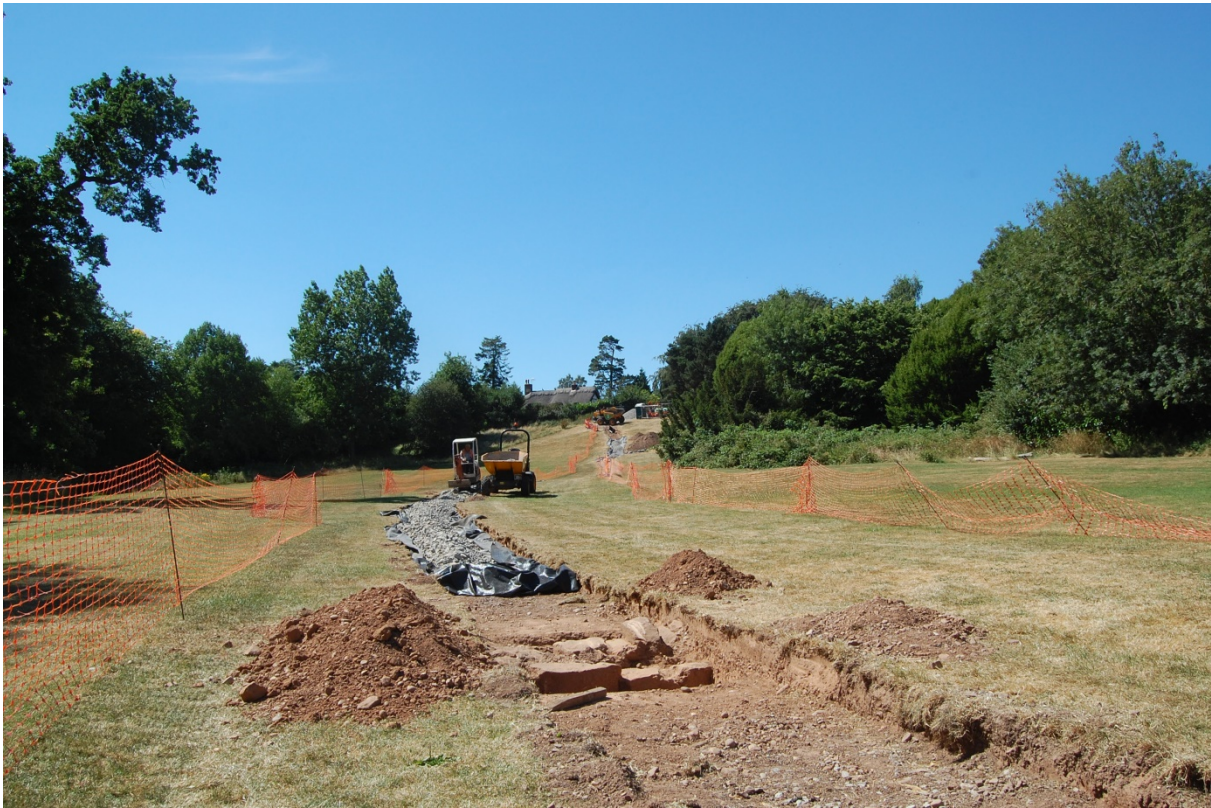
13: North-west-facing view of site with wall 109 in the foreground and positioning of foundation material for new path in progress beyond
