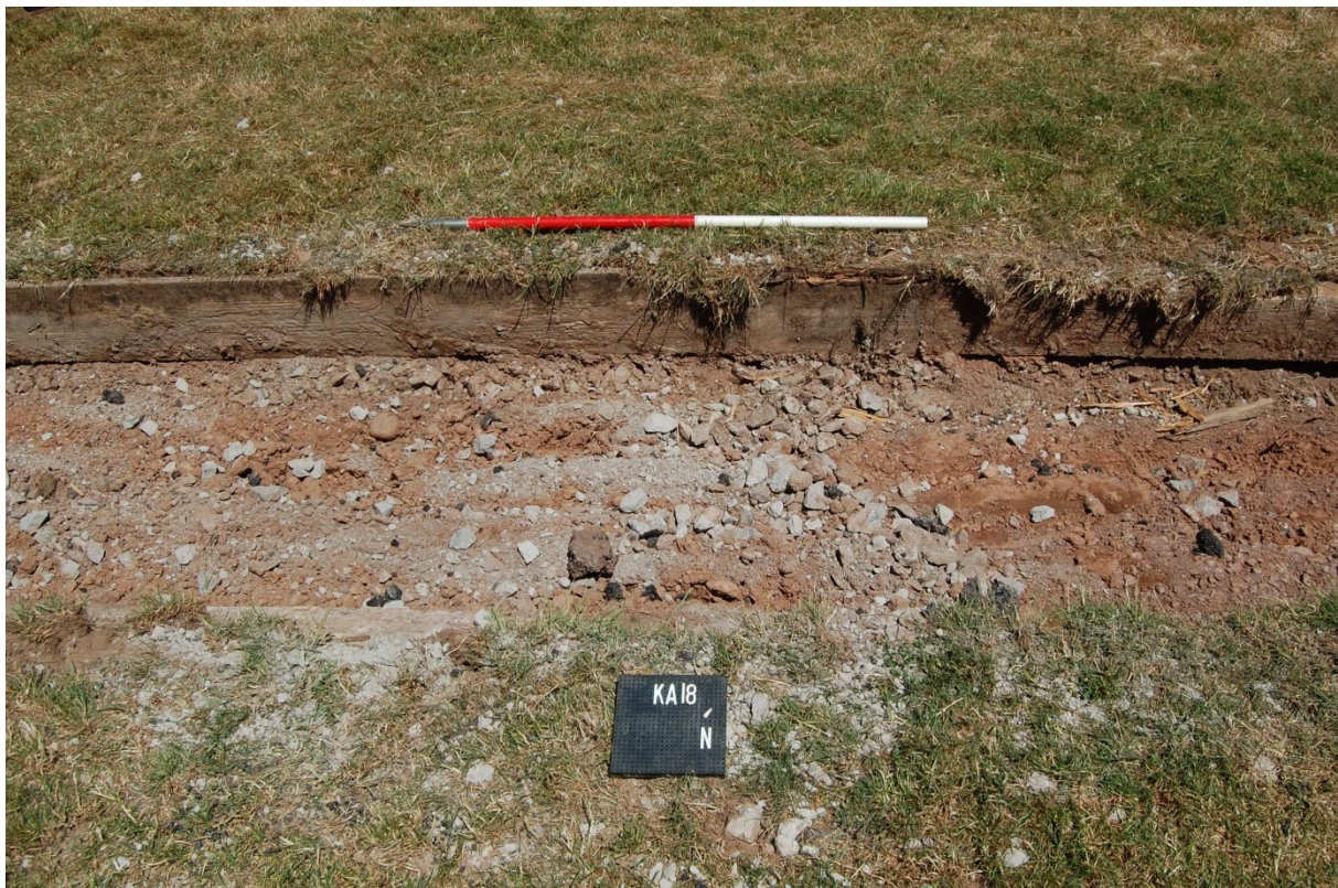
22: Trench for new footpath following removal of modern tarmac, looking north-east, showing the wooden boards either side of the existing path
